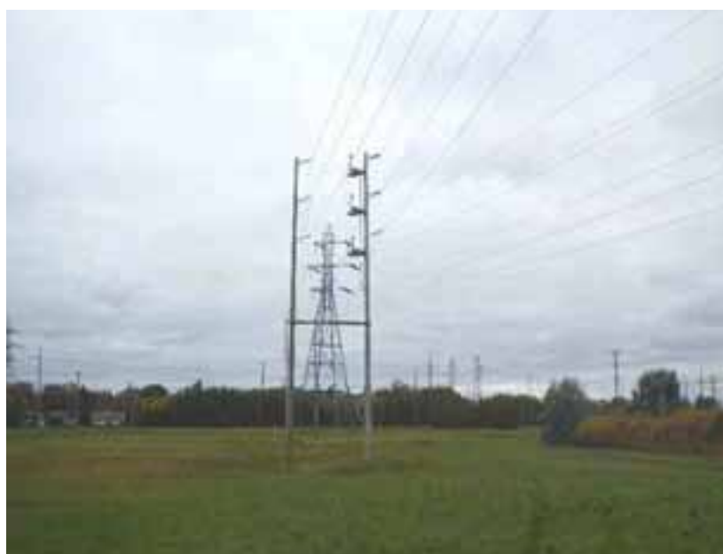
Figure 4: Existing overhead electrical infrastructure – looking south through the Parker Lands (mid site).
